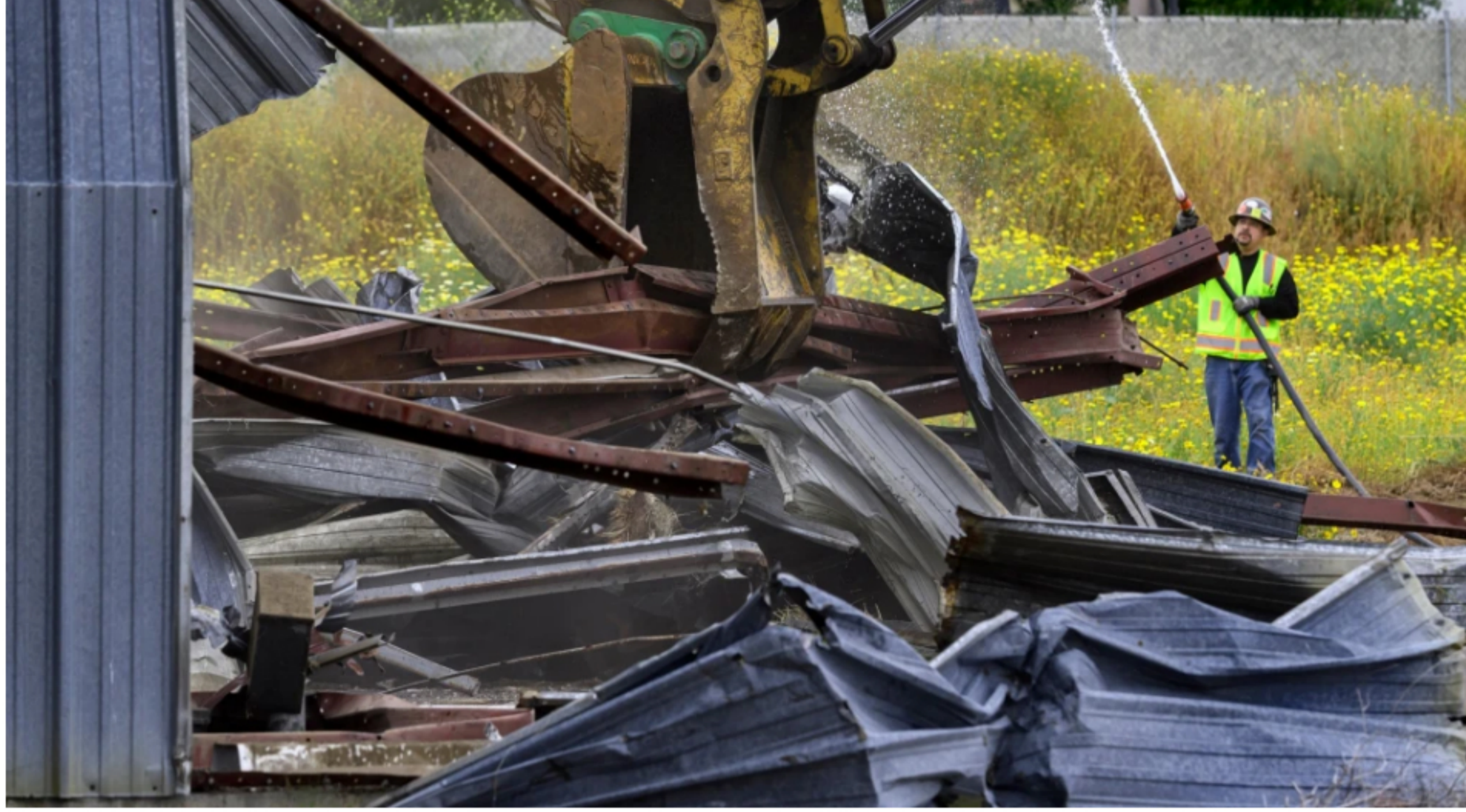
A demolition crew takes down a building, circa early 1970s, that stored air compressors at the former El Toro Marine base in Irvine on Tuesday, May 23, 2023. The city celebrated the next phase of the Great Park development with a groundbreaking. The $1 billion project will develop 1,300 acres and have a park twice as big as Central Park in New York. City Councilman and Chairman of the Great Park Board, Mike Carroll, said. (Photo by Mindy Schauer, Orange County Register/SCNG)
