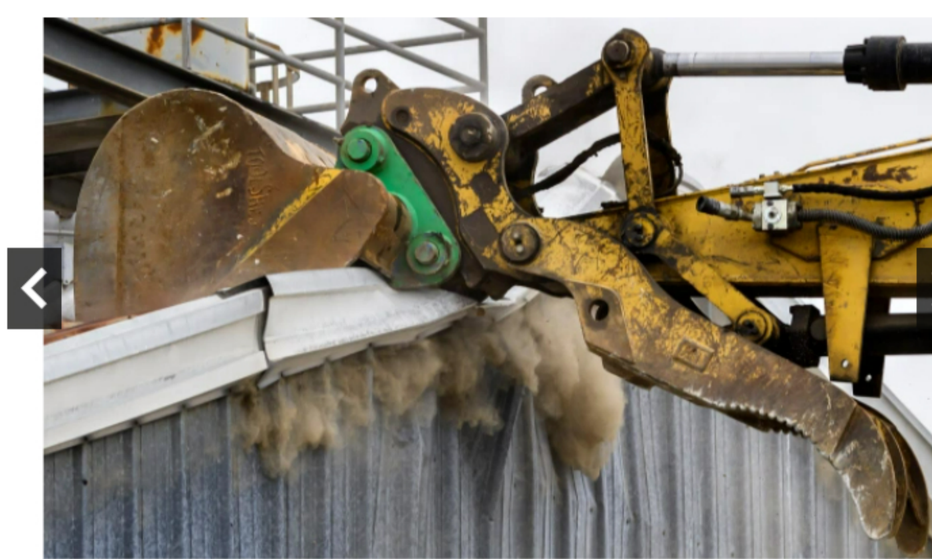
1 of 10 A demolition crew takes the first chunk out of an early 1970s-era building that stored air compressors at the former El Toro Marine base in Irvine on Tuesday, May 23, 2023. The city celebrated the next phase of the Great Park development with a groundbreaking. The $1 billion project will develop 1,300 acres and have a park twice as big as Central Park in New York. City Councilman and Chairman of the Great Park Board, Mike Carroll, said. (Photo by Mindy Schauer, Orange County Register/SCNG)
