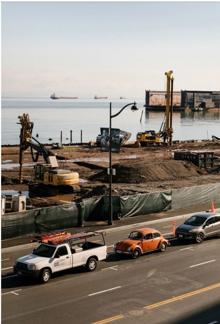
A public park being built across Terry A. Francois Boulevard. Jason Henry for The New York Times
